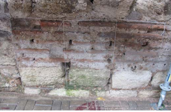
Picture 30. Controlled sandblasting examples on the façade, aluminum oxide, dolomite and apricot skin
