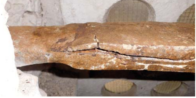
Picture 41. Beyazıt Mosque main dome broken reinforcement detail (2013)
