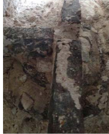
Picture 38. Azapkapı Sokullu Mehmet Paşa Mosque, metal tie rods with ring supports reinforcement detail. 2014
