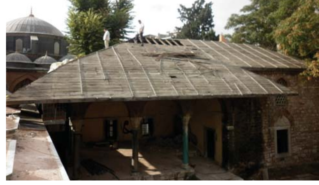
Picture 5. The relation of the roof of Infants' School with the domes of madrasah (E. Sünnetçi, 2010)
