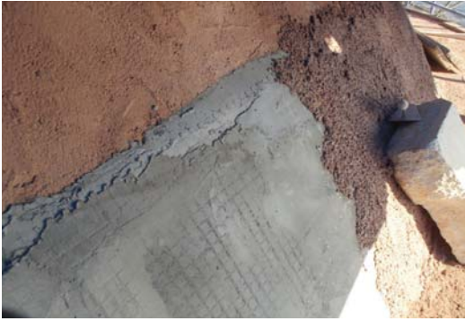
Picture 27. Fibrous polymer straw mesh reinforced mortar implementation stages (Fındıklı Molla Çelebi Mosque – 2014)
