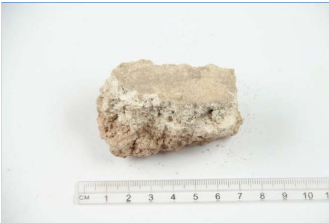
Picture 2. Render and smoothing sample that has been taken from the external façade
