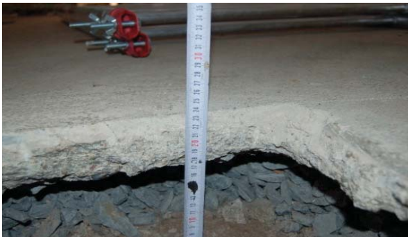
Picture 49. Concrete and blockage embankment on the masjid floor Resim 49. Mescit zeminindeki beton ve blokaj dolgu
