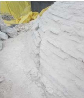
Picture 6. K1 dome crack detail – Internal view (2013)
