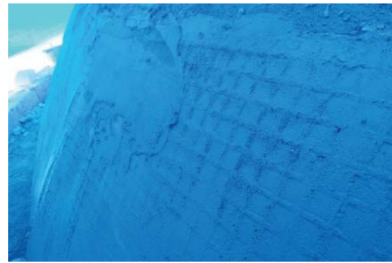
Picture 25. Fibrous polymer straw mesh reinforced mortar implementation stages (Fındıklı Molla Çelebi Mosque – 2014)
