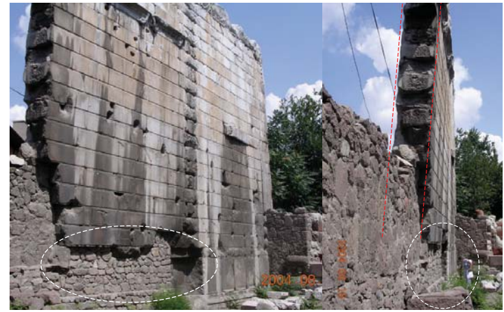
Picture 1. Damaged and inclined north wall of the Augustus Temple
