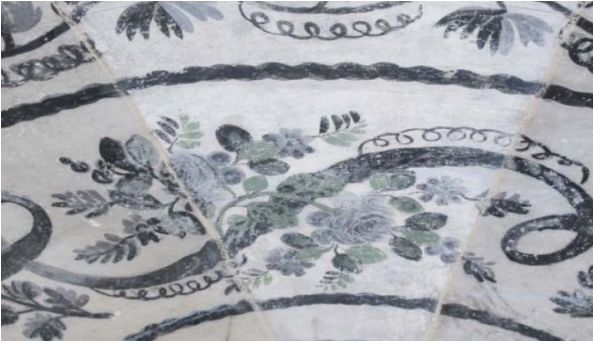
Picture 45. As a result of the scraping of the existing dome adornment, it is seen that the composition of the adornment beneath is the same, except color was used in some places
