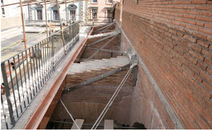
Picture 3. View of the southern lateral longer side of the Great Vault with the diagonally counterbraced shear reinforcements placed in the free spaces between the Vault itself and the Southern building, nearly the ending of the work.
