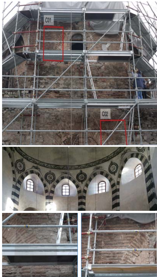
Picture 7-12. Work phases and overview of the Masjid when the restoration has been finished
