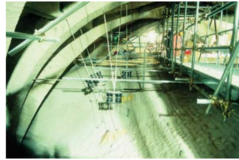
Picture 20. The Basilica of St. Francis in Assisi: The provisional "flying bridge" suspended to the roof
