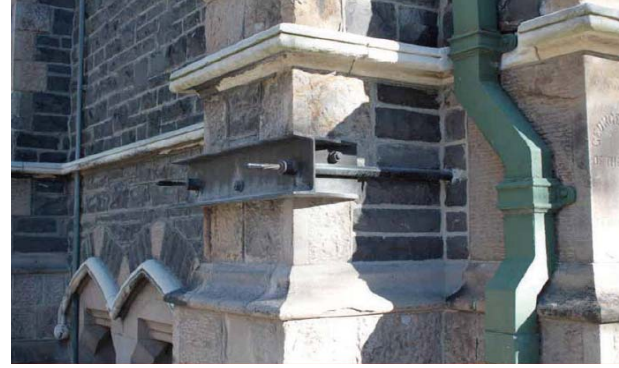
Picture 3. Old strengthening technique: Steel/Iron cerclage, masonry building in Christchurch, New Zealand
