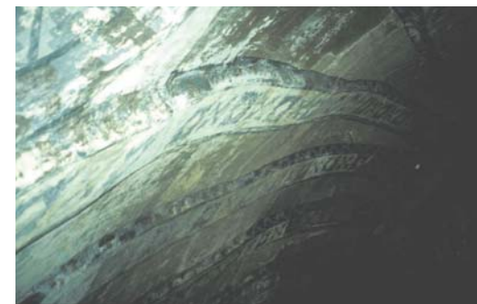
Picture 13. Hagia Sophia: Large deformations on the ribs
