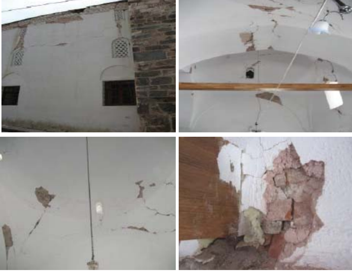
Picture 2. Damages Occurred in Great Mosque
