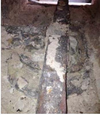
Picture 39. Azapkapı Sokullu Mehmet Paşa Mosque, metal tie rods with ring supports reinforcement detail. (2014)
