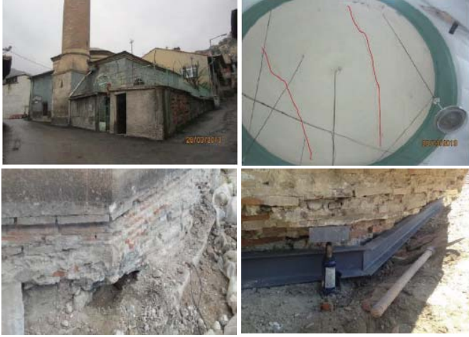
Picture 11. Dome damage of Kurşunlu Mosque in Kütahya
